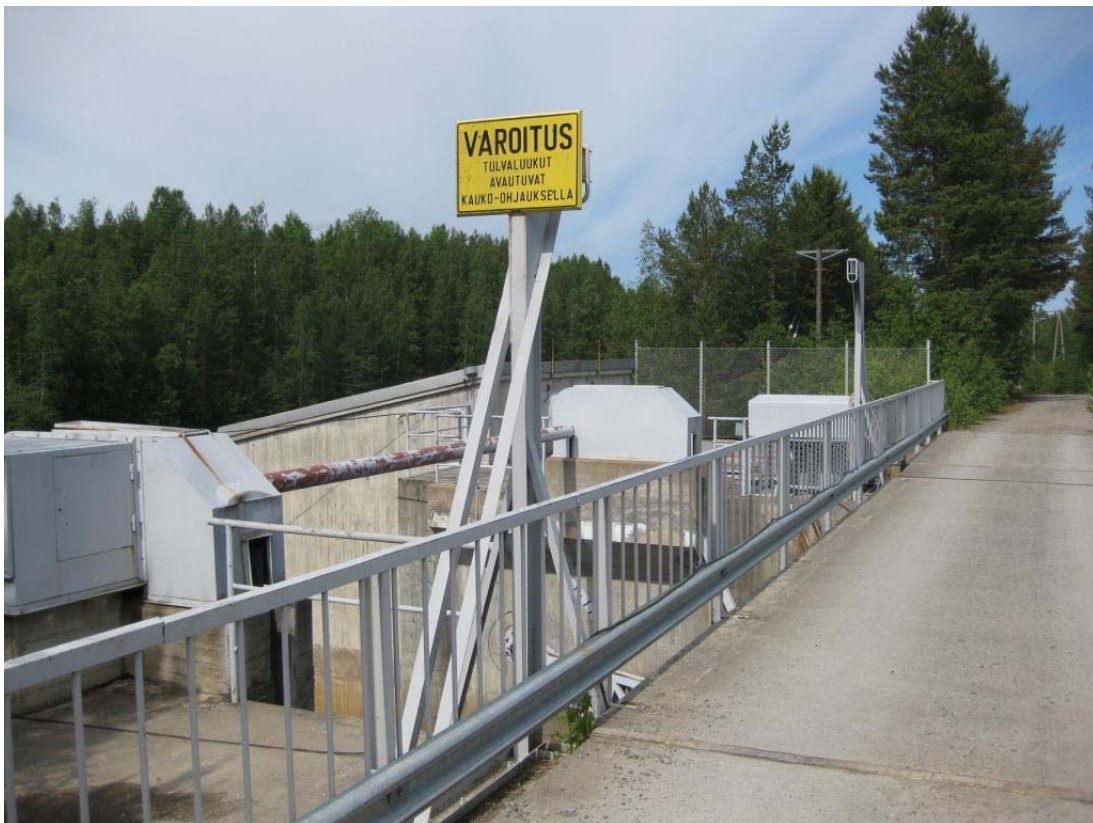
Figure 3. Safety arrangements i.e. signs, fences, rails, the arrangements of the gate openings (e.g. sirens) and the risks were reviewed during the site visits.
