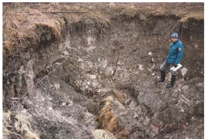
Figure 4: A large sink hole was formed due to the internal erosion in 1987.
