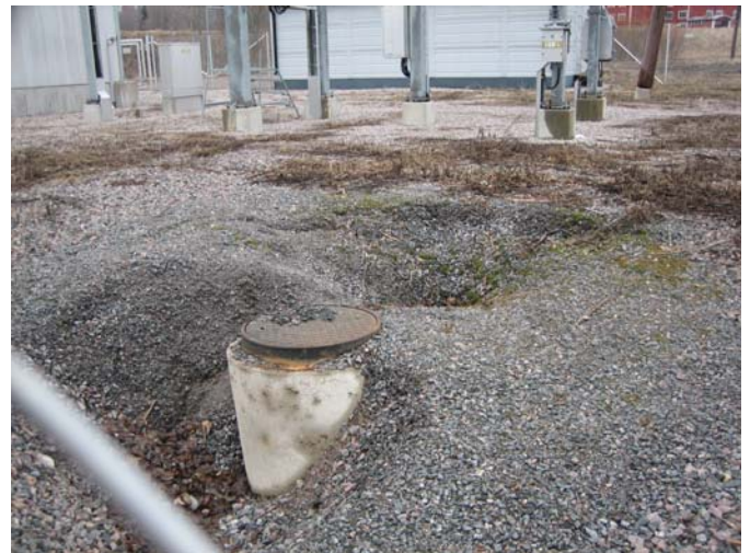
Figure 7: The sink holes at the substation on March 21, 2007.
